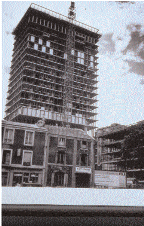
É. Albert, tour Croulebarbe, Paris, 1956-1961, chantier (source: Archives Albert, Mnam-Cci, Centre Pompidou)
